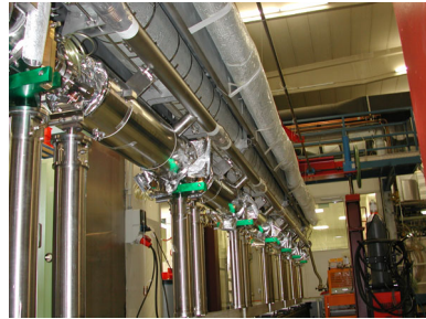
Cavity string connected
