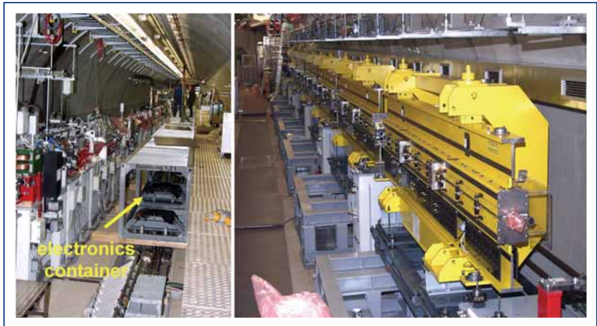
Figure 2.3.2 Left: FLASH accelerator tunnel with part of the collimator section and an electronics container visible. Right: The undulator consists of six segments, each 4.5 m long.
