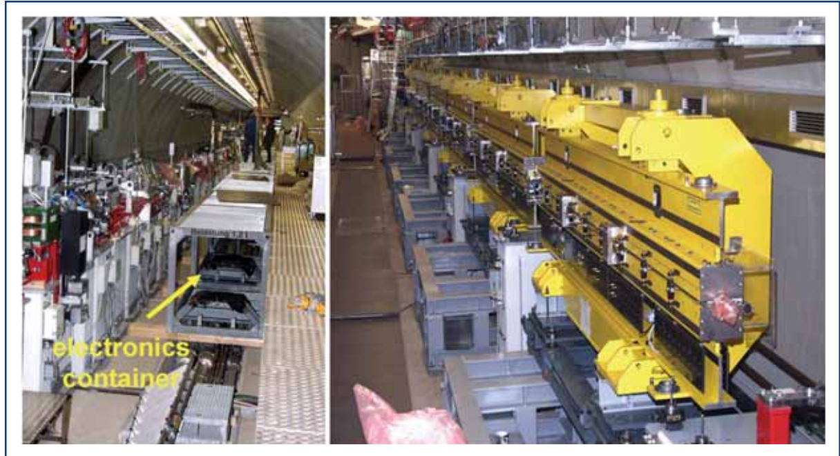
Figure 2.3.2 Left: FLASH accelerator tunnel with part of the collimator section and an electronics container visible. Right: The undulator consists of six segments, each 4.5 m long.
